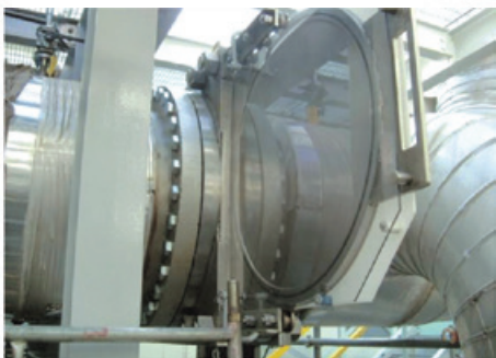
Heat exchanger - Bypass line
