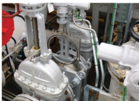
JET - Fuel (MOV automation)
