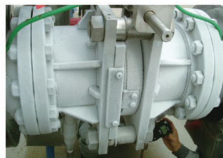
Cryogenic service (LNG / Ethylene)
